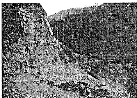
Large scale slope failure on provincial highway in NWFP, Shinkiarai - Nawaz Abad Road in Mansehra District
